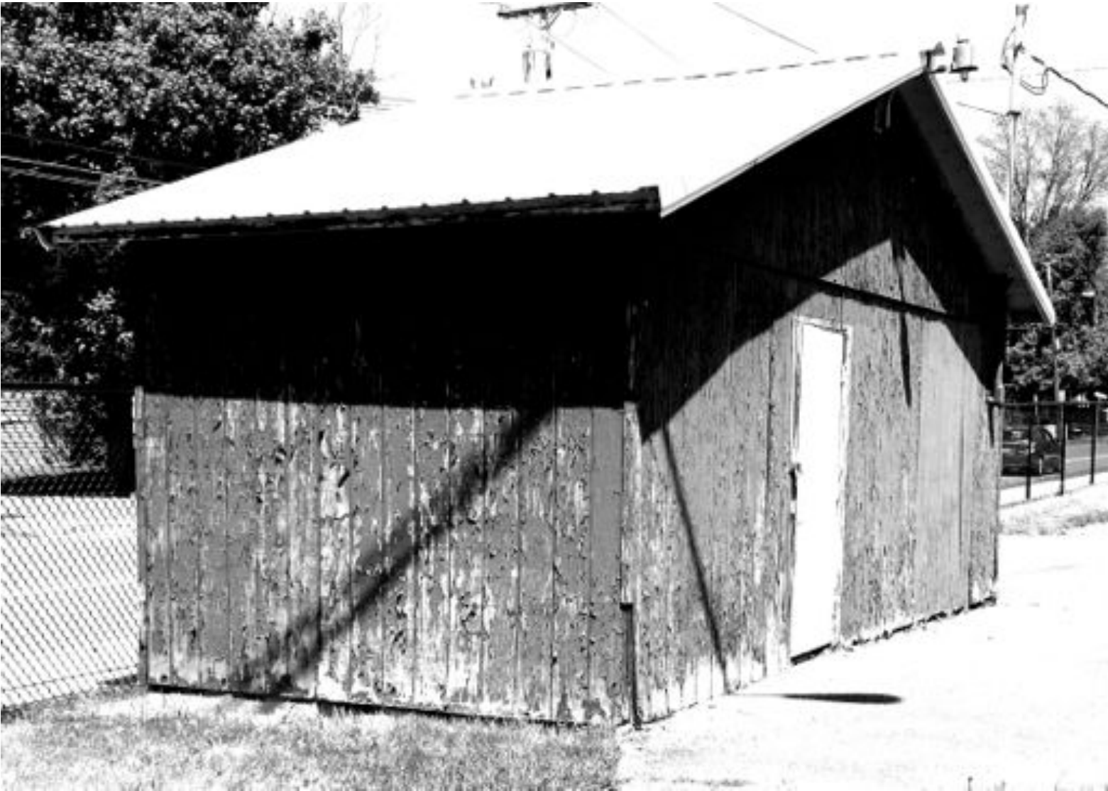
Arts and Crafts Shed. Floral Ave. Park, Johnson City (Note peeling paint etc. Plywood may be better. Also close fence)
